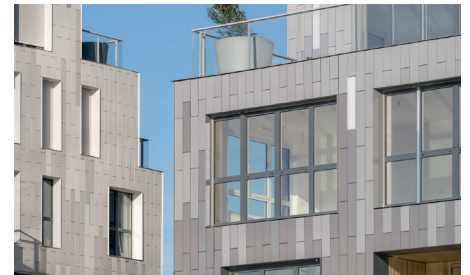
The buildings consistently mix social housing and condominiums, large and smaller flats with dual and triple orientations.
